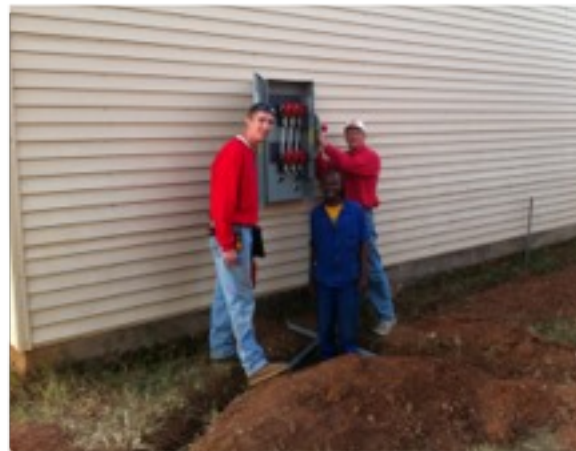
To allow for the new surgical center, the entire electrical system on the campus was redesigned & shipped from America. Many thanks to Crosby Electric in Montgomery, AL who donated supplies and one of their technicians!
